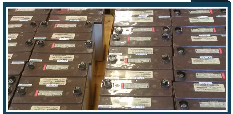
Previous Battery Strings in TTC's Data Center
