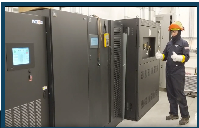
VYCON's VDC Flywheel paired with 3-phase Double-Conversion UPS system.
