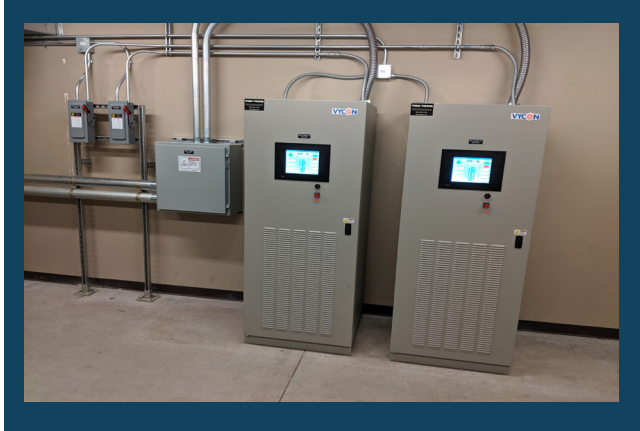
VYCON VDC-XXT 450kW flywheel systems
