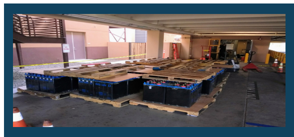
Wet cell batteries located in the garage.
